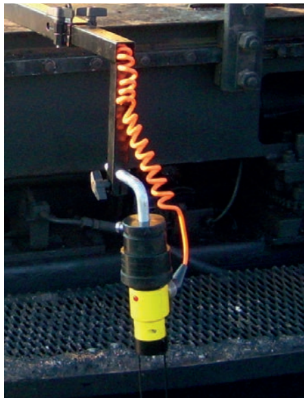
The sensors are connected by the internal cabling of the Averaging Beam.
