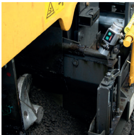
Mounting of the AC700 at the auger
